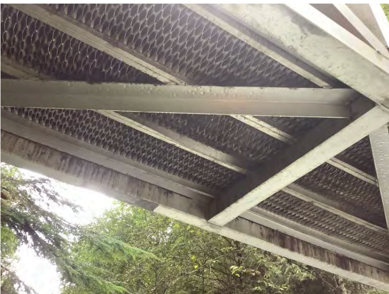
Deck - underside of deck torn. Planks above support live loads now
